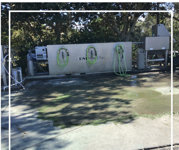
Closed loop systems provide not only protection against discharge of nutrient rich wash water but also help conserve water.
