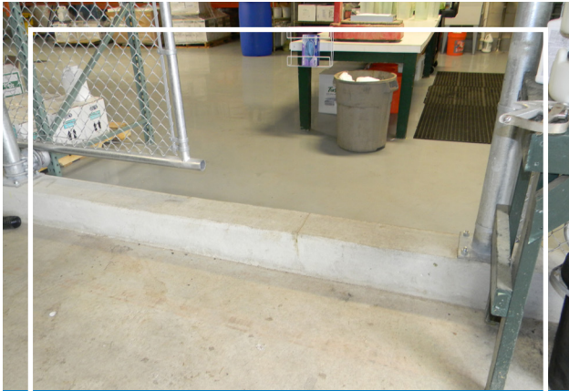
Design features like raised curbing can provide containment in case of a chemical spill.
